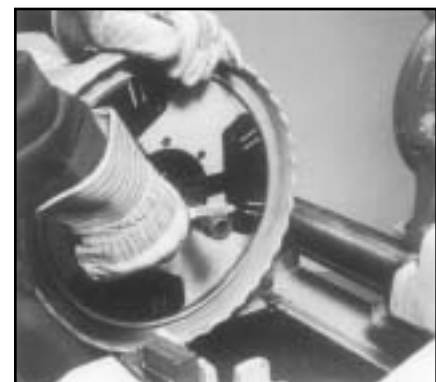
Figure 16: Using a utility knife to "pencil-cut" PVC coating before threading conduit. (Courtesy of ROBROY Industries Conduit Division)
